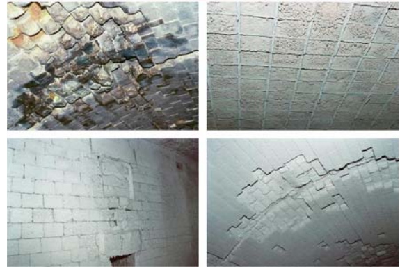
Figure 4 – Tunnel kiln refractories that have been coated with EMISSHIELD®.
